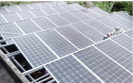
Power supply for Son Cha island – Hue Capacity: 10 kw Off-Grid Pv
