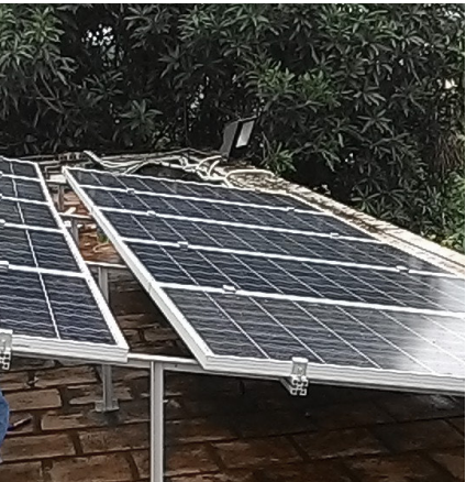
Mr. Vương's house - Dist. Hoang Mai - Hanoi Capacity 2kWp - Installed in Sep 2015
