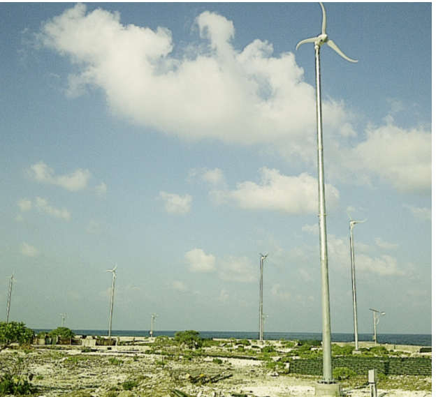
Project Guesshome in Southwest Cay Island (Song Tu Tay) – Trương Sa. Capacity: 06 wind turbines Skystream 3.7 with 14,4kW in total.
