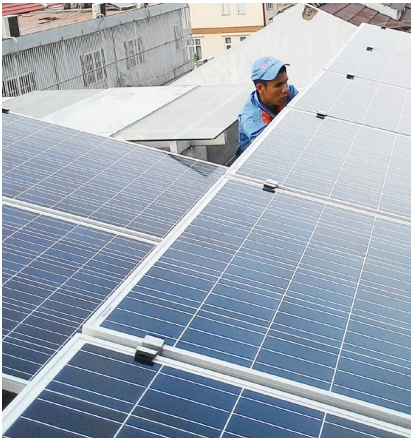
Mr. Thanh's house - Dist. 7 - HCMC Capacity 2kWp - Installed in May 2015
