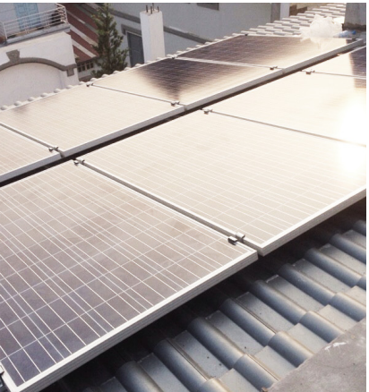
Mr. Quân's house - Dist. 2 - HCMC Capacity 2kWp - Installed in Oct 2015
