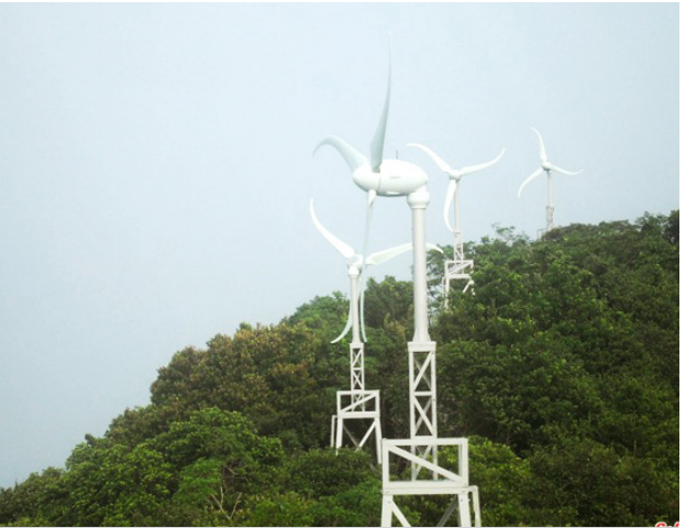
Project Trần-Quân Area 3, Quảng Ninh. Capacity: 5 wind turbines Skystream 3.7 with 14,4kW in total and PV
