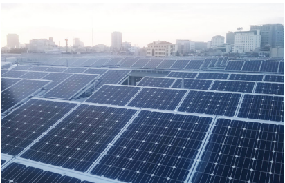
Green One UN Home in Vietnam. Capacity: 110kWp
